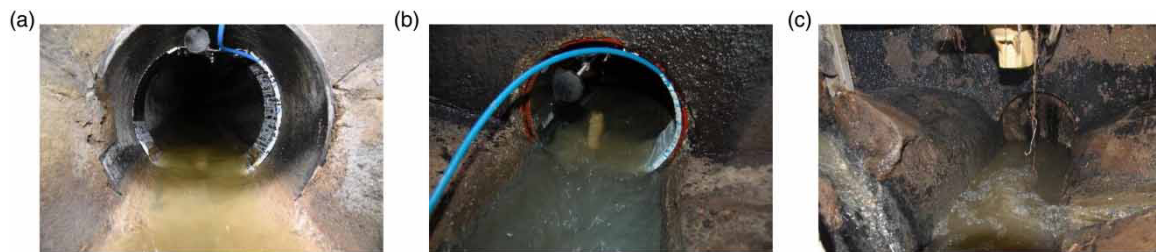
Figure 6 | Examples of sensors poorly installed in sewers. (a) Sensor in a supporting ring, top of the pipe (b) Sensor in a supporting ring, bottom of the pipe (c) Sensor above the pipe, in the manhole wall.
