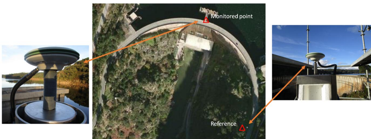
Fig. 2 – GNSS system installed in Cabril dam for measure the displacement at the top of central section
