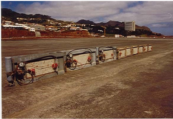
Figure 9. The creep and shrinkage compensator in situ
