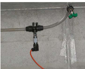
Fig. 4 Pressure cell used in hydrostatic levelling system
