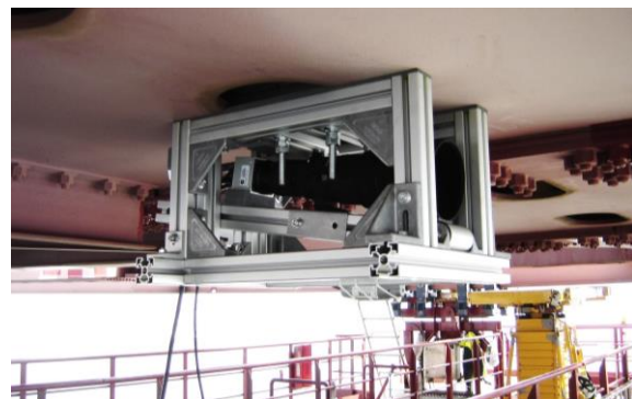
Figure 5. Camera installed in the P25A suspension bridge main span central section.
