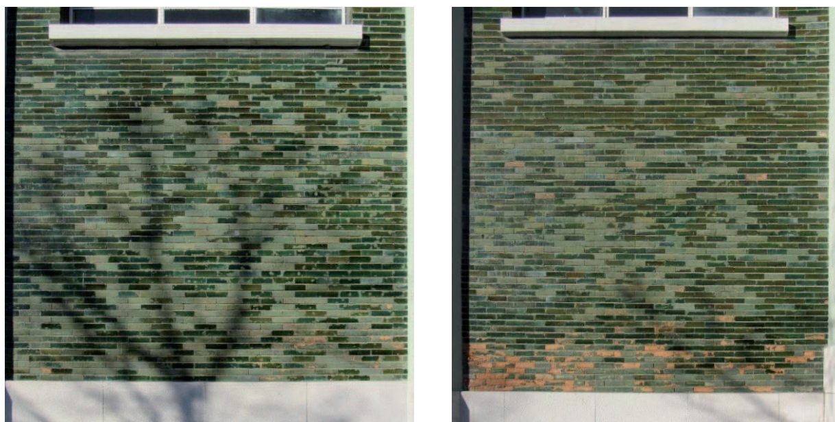
Figure 4: Casa da Moeda, Lisbon. Left: preserved as originally; right: decayed at bottom
