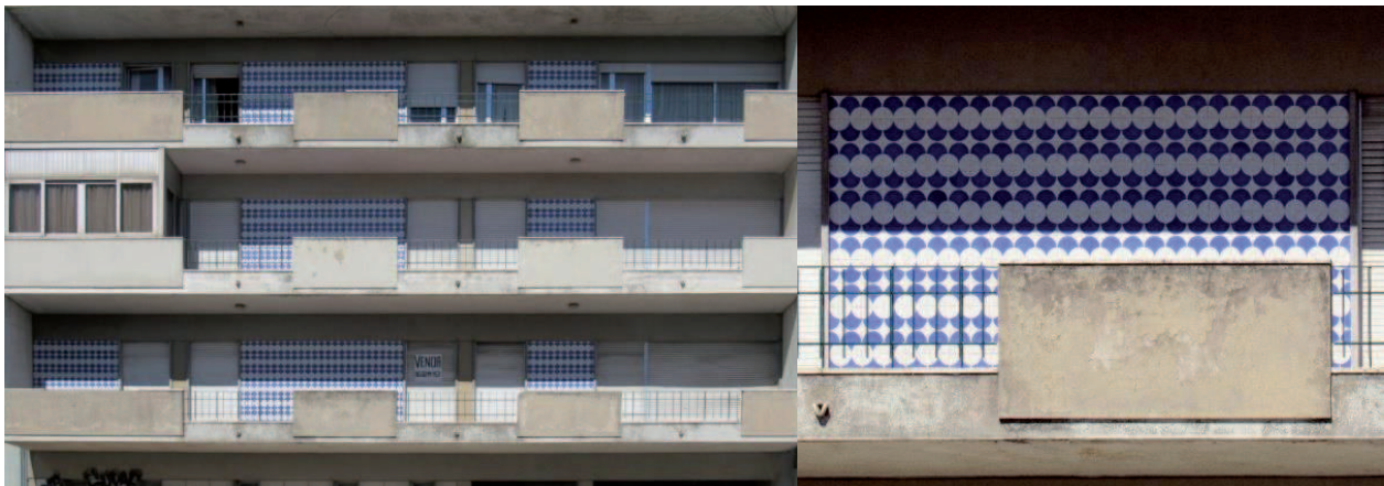
Figure 2: Repetitive pattern mostly hidden from a street view. Avenida Rainha Dona Amélia Nº 52, Lisbon
