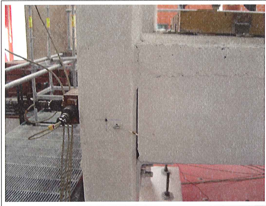
Figure F-17: Detail of the beam-column connection after stage 02 (J6-Trans.)
