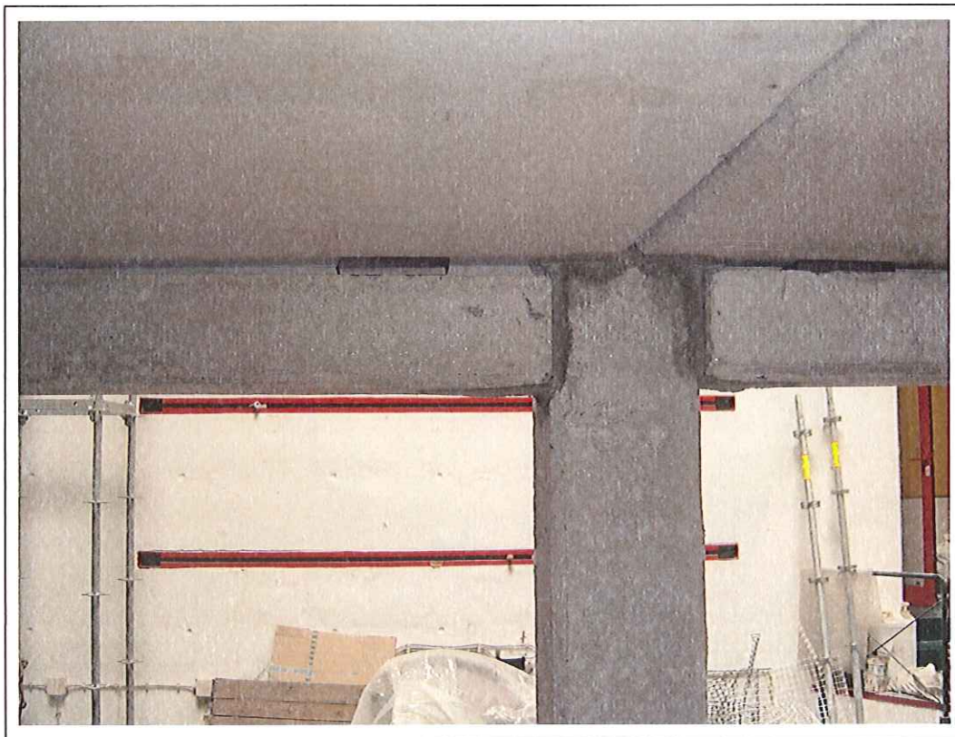
Figure F-6: Detail of the contact points between the slabs and the longitudinal beams
