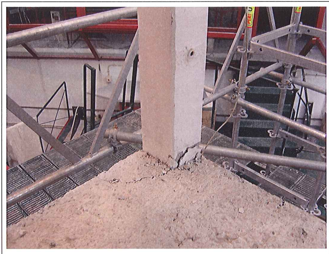
Figure F-36: Detail of cracking on the topping layer (J1)
