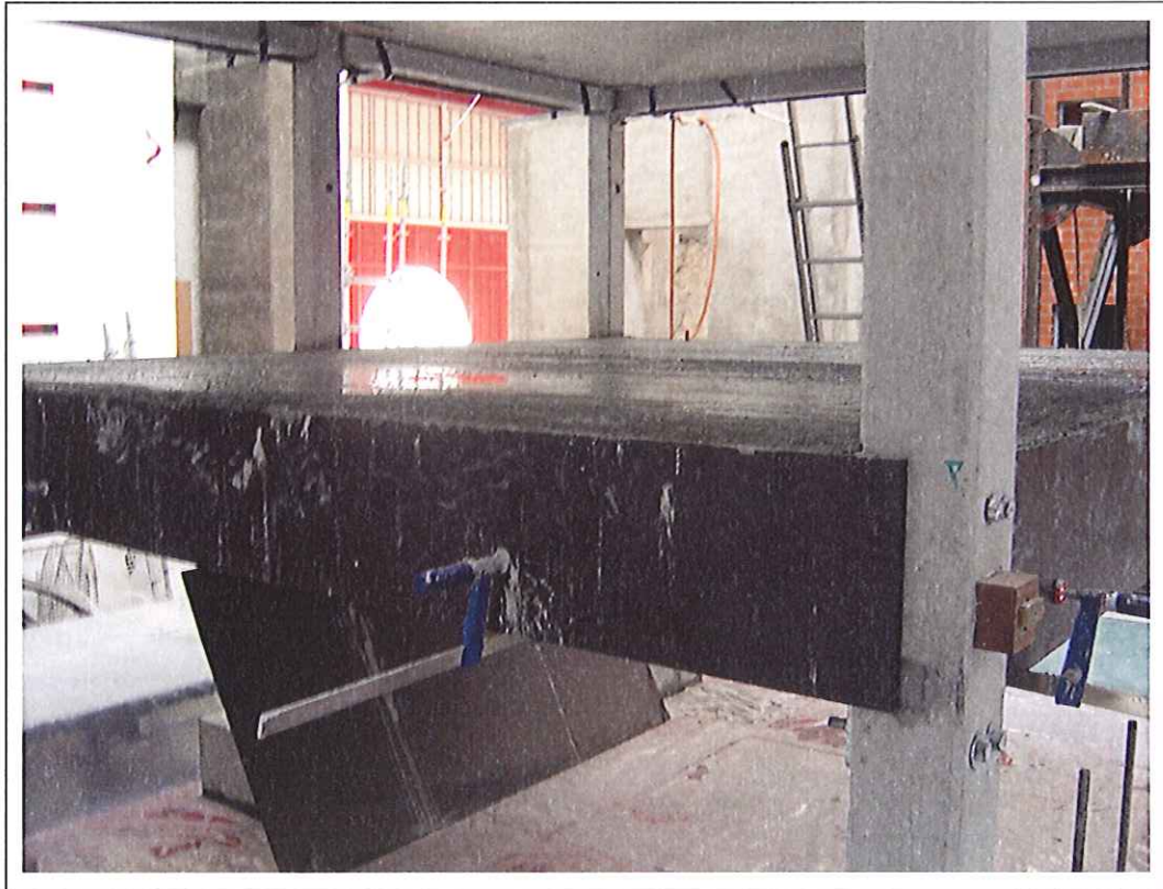
Figure F-8: General view of the first floor slab after concreting the topping layer
