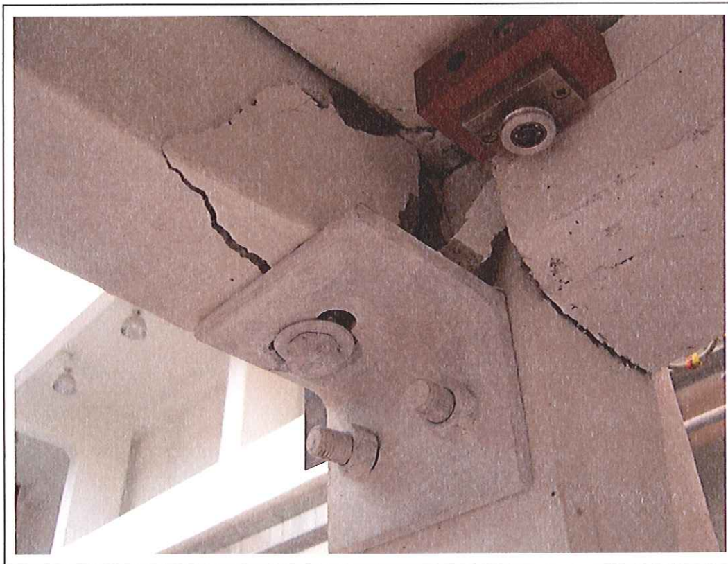
Figure F-22: Detail of the beam-column connection's inner part after the test (J9-Trans.)
