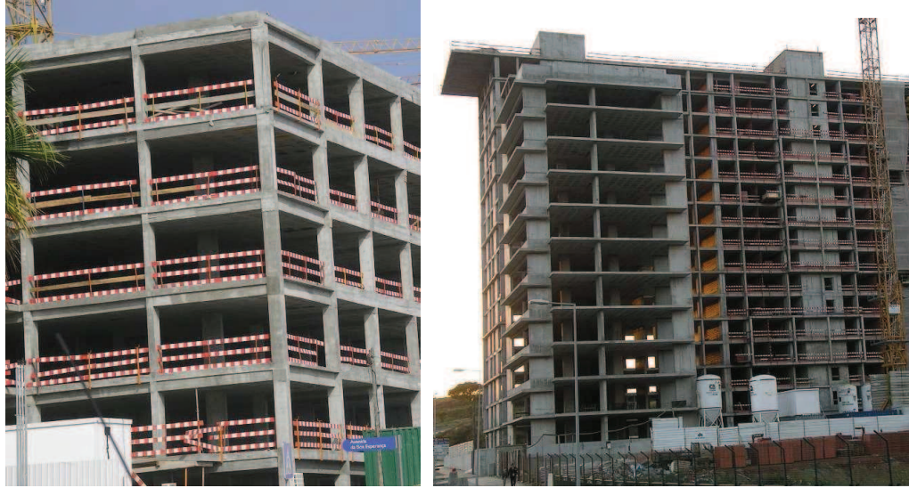
Figure 3.9 – RC buildings constructed after RSA code being enforce. Left: RC frame building; Right: RC dual systems [after Sousa, 2005].
