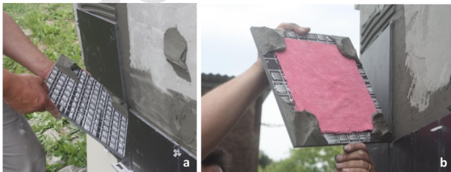
Fig. 2. Simulation of the anomalies of detachment (a) and placement of the water absorptive cloth beneath a tile (b).
