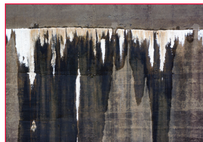
Figure 27: Flight A. Central crack photographed with a focal length of 50 mm
