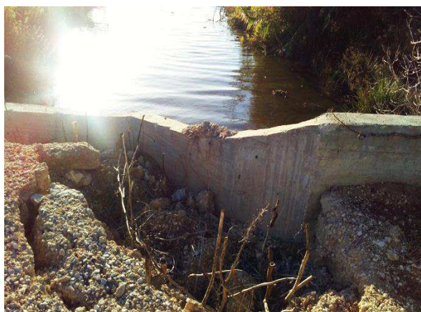
Figure 2.10 – Example of internal erosions a few kilometers downstream of site 10 (November 26, 2015)
