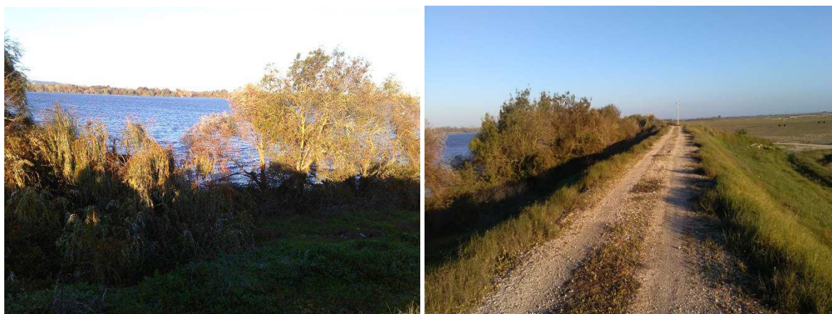
Figure 2.11 – Site 10: Area of the dyke break during the fluvial flood of 1979 (November 26, 2015)
