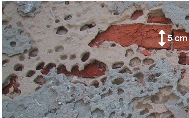
Fig. 5 - Alveolar decay of salt-hardened lime plaster with cement repairs, on an old building façade at a coastal area near Lisbon, Portugal
