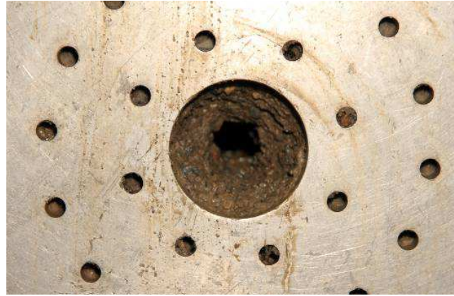
(d) After removal of retained material. Hole was not filled with material eroded from upstream.
