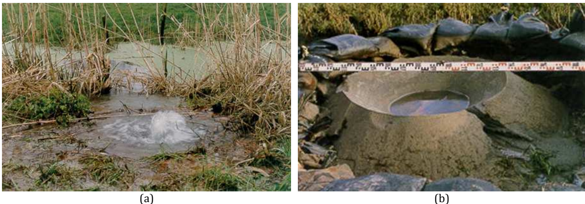
Figure 2.3 – (a) Sand boil at downstream of the toe of the embankment; (b) Small dam of sand bags around sand boil (Sellmeijer and Koelewijn, 2007).
