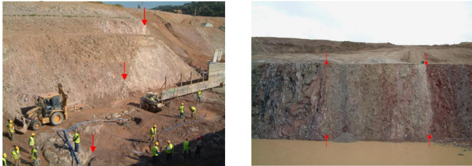
Figure 4: Fault zones crossed by the geophysical profiles. Left - zone A on Figure 3. Right - the downstream limit (point C ) of the fault zone B-C on Figure 3 8 .
