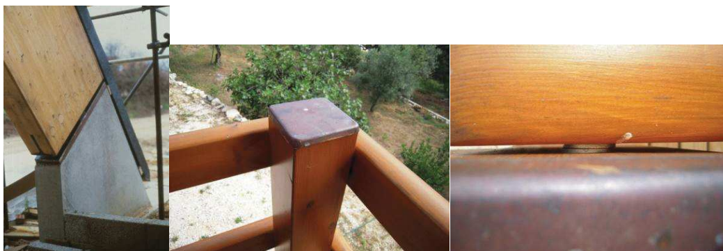
Figure 2. Timber resting on a concrete column to avoid contact with ground water; metal cap of the column end-grain surface; washers to space contact surfaces (top view)
