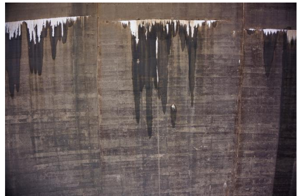
Figure 28 – Flight B. Central crack photographed with a focal length of 16 mm.
