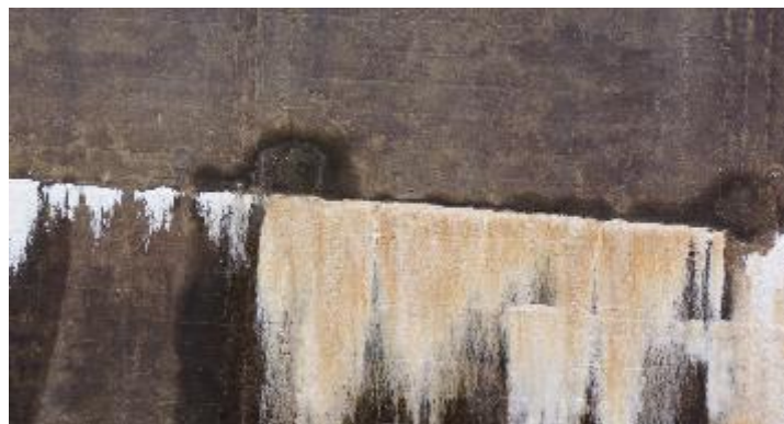
Figure 10: A detail of crack n.º 3 (crack on the right side).
