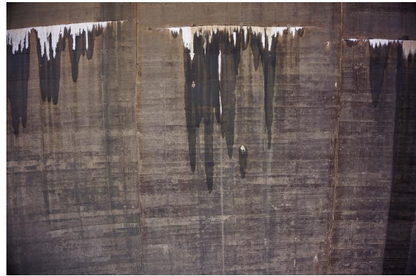
Figure 8: Flight B. Crack n.º2 (between cracks n.º1 and n.º3) photographed with a focal length of 16 mm.
