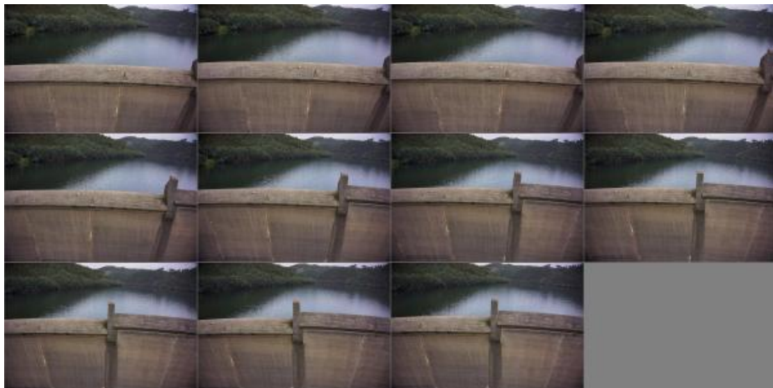
Figure 18: Photos used to generate the 3D model (point cloud) of the spillway.
