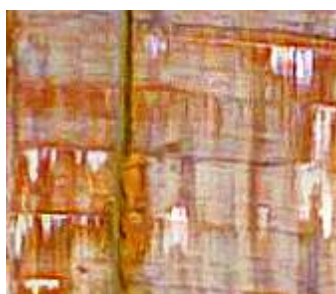
Figure 6: Photo of the downstream face with colour enhancement.
