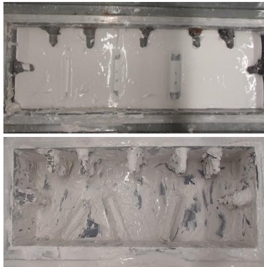
Figure 6. Aspect of the pipes at the beginning (top) and at the end (bottom) of the preliminary tests.
