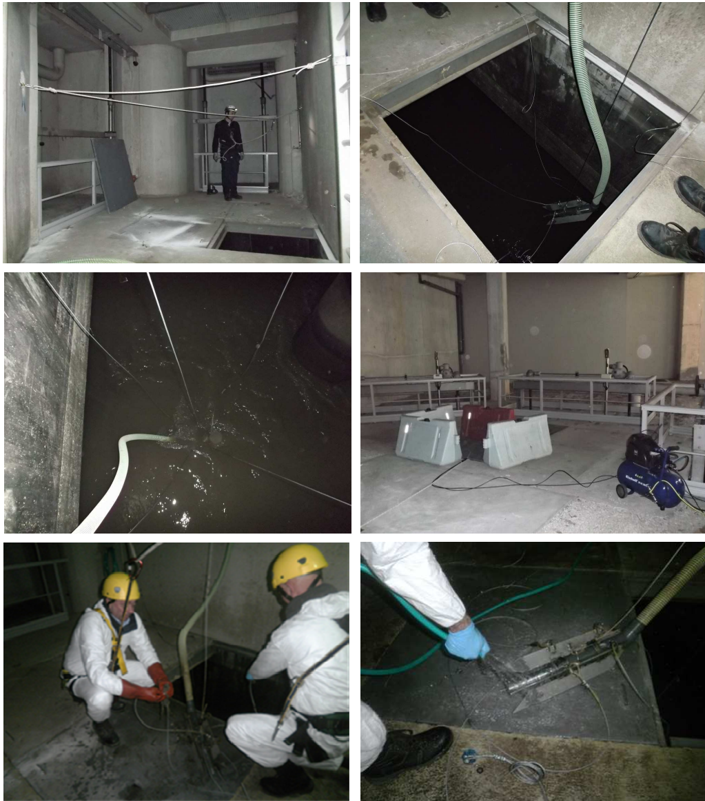
Figure 6 - Sewer on-line monitoring station: sensor installation and maintenance.
