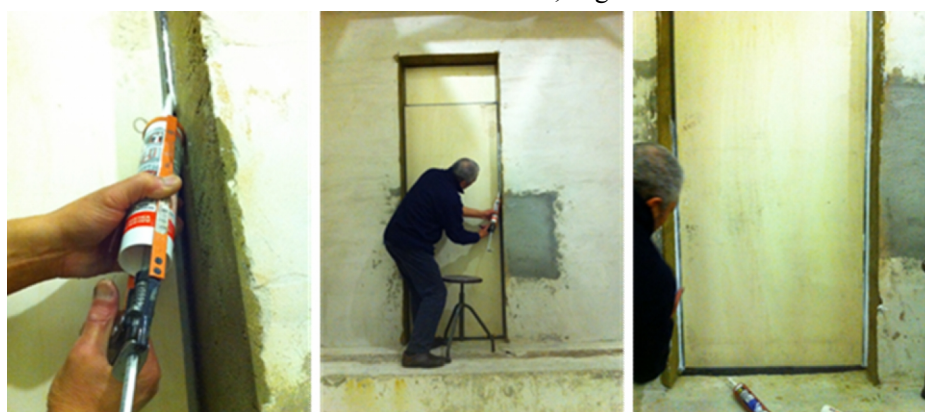
Figure 3 – Application of silicone in the gap between the sample and the opening.
