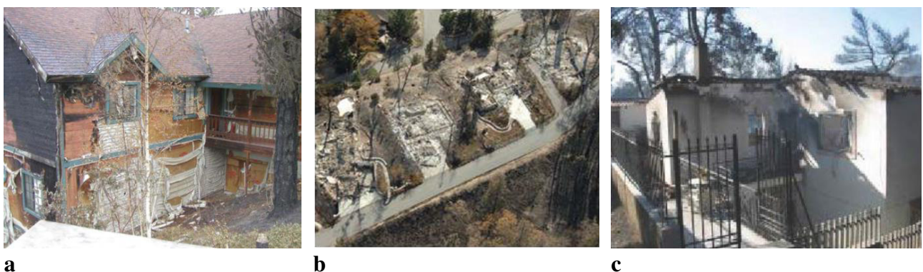
Figure 1. Influence of the construction materials characteristics on building vulnerabilities to wildland fire threats: a) building envelope damage due to the combustible construction materials (U.S.A.) (Cohen and Stratton, 2008); b) buildings destruction due to house-to-house fire spread (U.S.A.) (Cohen and Stratton, 2008); and c) building destruction due to its combustible contents (Greece) (Xanthopoulos et al. , 2011).
