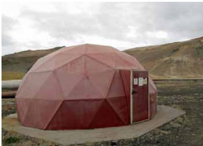
Figure 4 - Silencer in the borehole of the Krafla geothermal power (Iceland). Photo by Keith Clark (2000).
