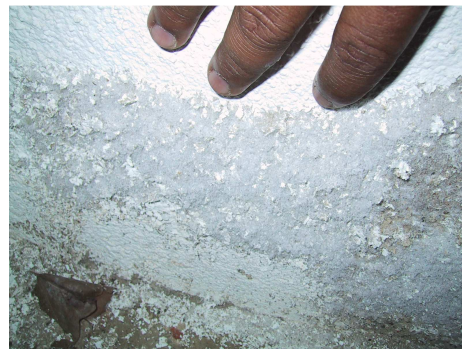
Fig. 9 - Efflorescences on the ground floor
