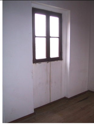
Fig. 18 - Water flow marks beneath a window of the mill first floor
