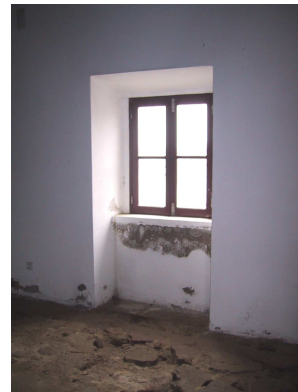
Fig.13 - Damaged (northern) wall and pavement of the mill ground floor
