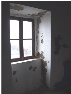
Fig. 12 - Peeling of the plastic paint around a northern window of the mill ground floor
