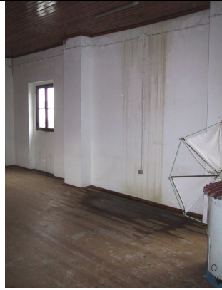
Fig.17 - Water flow marks coming from the ceiling, at the mill first floor
