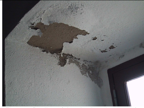
Fig. 11 - Peeling of the plastic paint around a northern window of the mill ground floor
