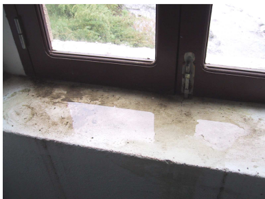
Fig. 14 - Puddles of liquid water – southern window on the mill ground floor
