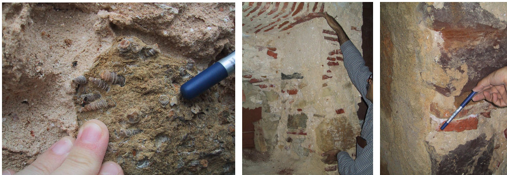
Fig. 19 - Masonry of the adjacent building: exterior (first at the left) and interior (two at the right)
