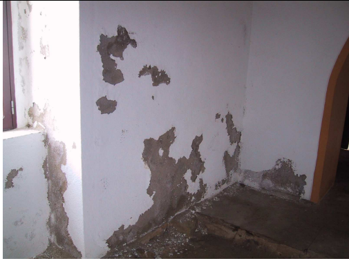
Fig. 10 - Damaged area of the mill N wall from
