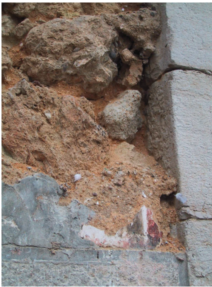
Fig. - Sanding and crumbling of the masonry bedding lime-mortars
