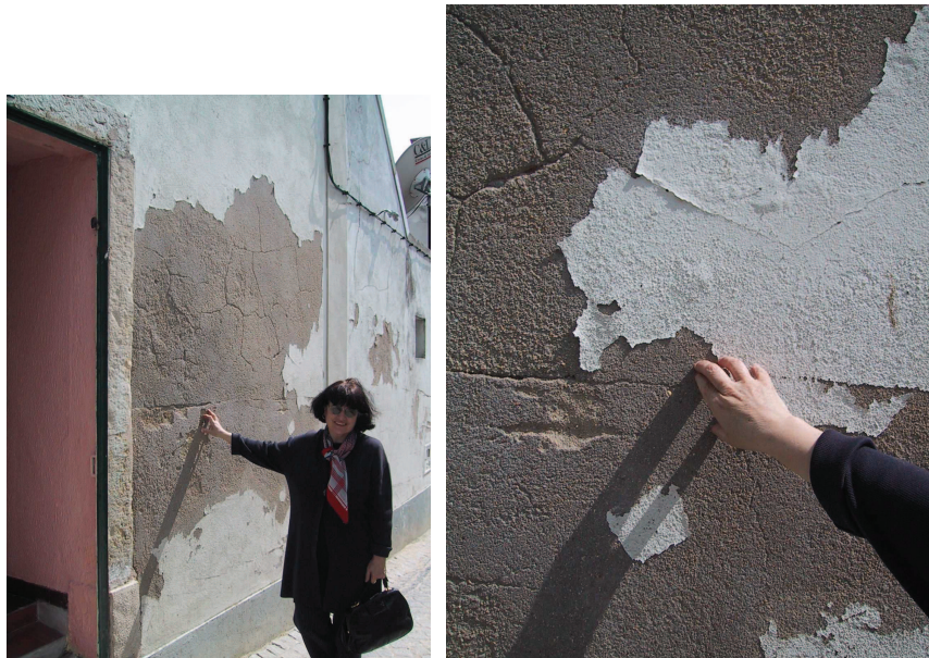
Fig. – Damaged building surfaces at ancient Almada (peeling of paints)
