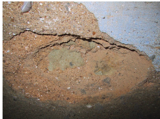
Fig. - Sanding and crumbling of the masonry bedding lime-mortars; detachment of a cement render repair
