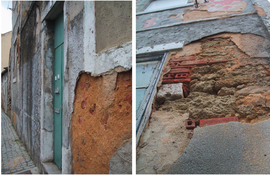
Fig. – Damaged building surfaces at ancient Almada (sanding and crumbling of lime-mortars; detachment of cement renders)
