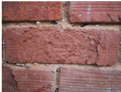
Fig. - Scaling of ceramic bricks at a masonry repair
