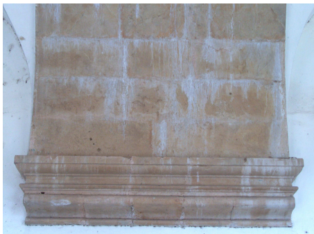
Fig. 13 – Efflorescences spread from the joints of stone elements (2003-11-27)
