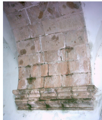
Fig. 14 – Efflorescences, moss and moisture spots on stone (2004-02-05)
