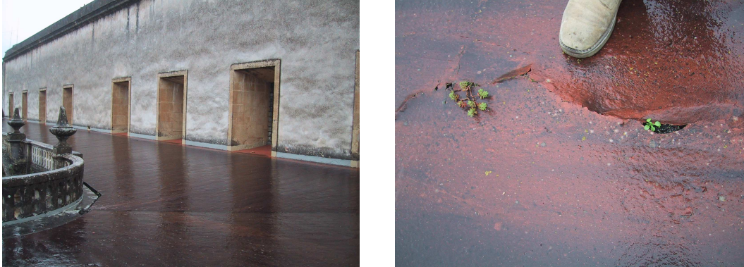
Fig. 19 – Damaged roof covering (2004-01-08)
