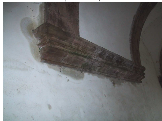
Fig. 10 – Moisture spots on the interface render / stone element (2004-01-08)
