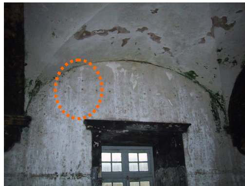
Fig. 20 – Infiltration of water from the rain through the roof and accumulation on the second floor pavement (2004-01-08)
