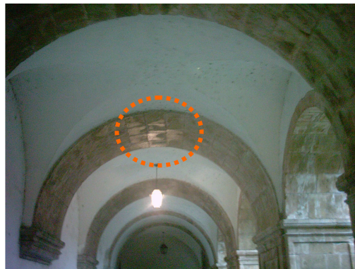
Fig. 21 – Liquid water on the vaults and pavement stones (2004-01-08)
