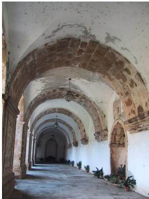
Fig. 7 - Cloister gallery: plaster damaged on vaults and moisture spots on stone (2004-02-05)
