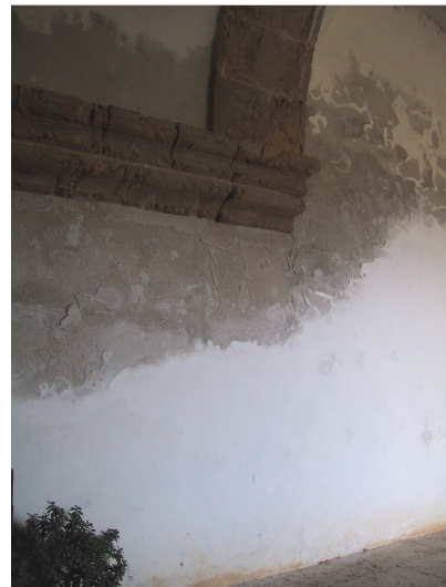
Fig. 8 - Cloister gallery: detail of a damage spot of the render/paint system, next to a stone element (2004-01-08)
