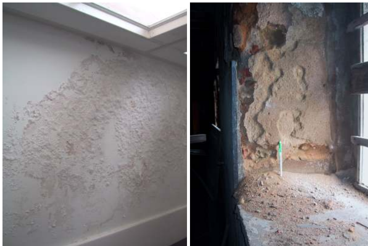
Fig. 1.1 - Two typical salt-damage patterns. Left: efflorescence and damage to paint, temporary exhibition gallery, south wing of Alcobaça Monastery, 2002. Right: sanding of lime plaster and of the lime bedding mortar leading to masonry disintegration, Paulistas tide-mill, Corroios, 2004.
