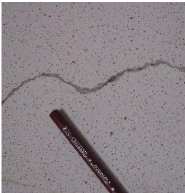
Fig. 6.17 – Sta. Clara: sporadic cracks are observed
