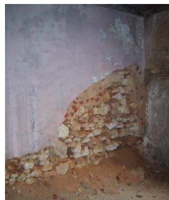
Fig. 2.4 - Masonry disintegration – Paulistas tide mill, Corroios, 2004
