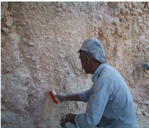
Fig. 6.32 – Before making the panels, the substrate was prepared as follows: (i) the old lime render, in poor condition and with many lacunas, was removed; (ii) the old lime mortar in the joints between masonry stones was removed up to a depth of around 15mm; (iii) the masonry was brushed to eliminate as much loose material as possible; (iv) all recesses deeper than 30 mm were filled with lime mortar A and small stones of the original masonry stone type.
