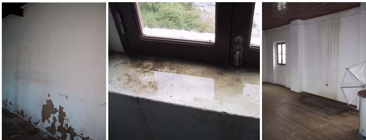
Fig. 6.9 – Tide-mill, damage on the southern wall. On the left: at the ground floor, salt damage appears mostly on the new hydraulic plaster. On the centre: lack of water tightness of the ground floor windows does not give rise to salt damage. On the right: infiltrations from the roof at the upper floor do not cause salt damage either.
