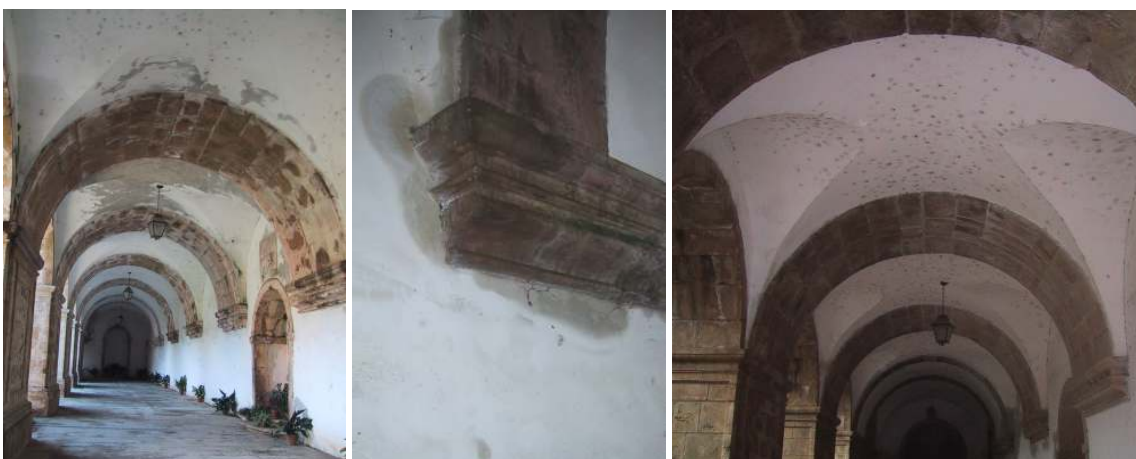
Fig. 6.19 – Sta. Clara: moisture spots on the stone (left), moisture spots and biological growth on the render (centre and right, respectively). On February 2004, on a sunny day that followed several cold rainy days, spots of liquid water were observed in the gallery, mainly on the surfaces of the stone columns and arches (left) with further absorption by the render (centre), which suggested the occurrence of dew point condensation. Biological growth is significant on the sheltered parts of the walls and vaults (right), which corroborates this hypothesis.
