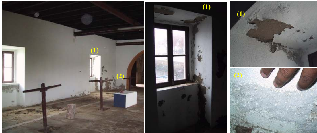
Fig. 6.8 – Tide-mill, damage at the northern wall of the milling room (ground floor). Left: general view showing that damage increases towards the N corner and appears mostly close to the ground or around the windows. Centre: peeling of the plastic paint around window. Right: damage to paint occurs either without (window frame in the top picture) or with (wall base in the bottom picture) efflorescence.
