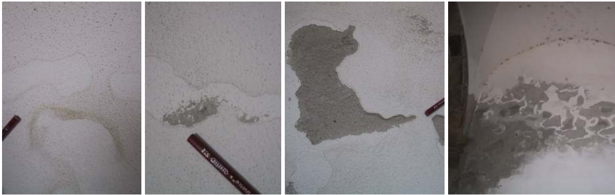
Fig. 6.16 – Sta. Clara: damage development. It is not known whether the borderlines between wet (darker) and dry (lighter) areas and, eventually, between damaged and non-damaged areas correspond to micro-cracks.
