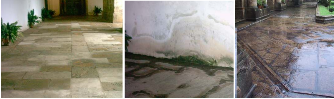
Fig. 6.20 – Sta. Clara: on the same day in February 2004 probable dew point condensation events were also observed on the stone floor (left and centre). Accumulation of water in the cloister garden (right) had been observed during a previous inspection, in January 2004.
