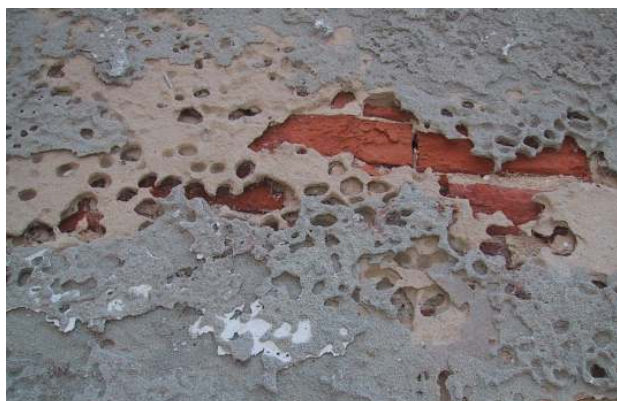
Fig. 2.3 - Alveolar decay – building adjacent to a branch of the Tagus river, at less than 10 km from the open sea, Alhos-Vedros, 2002
