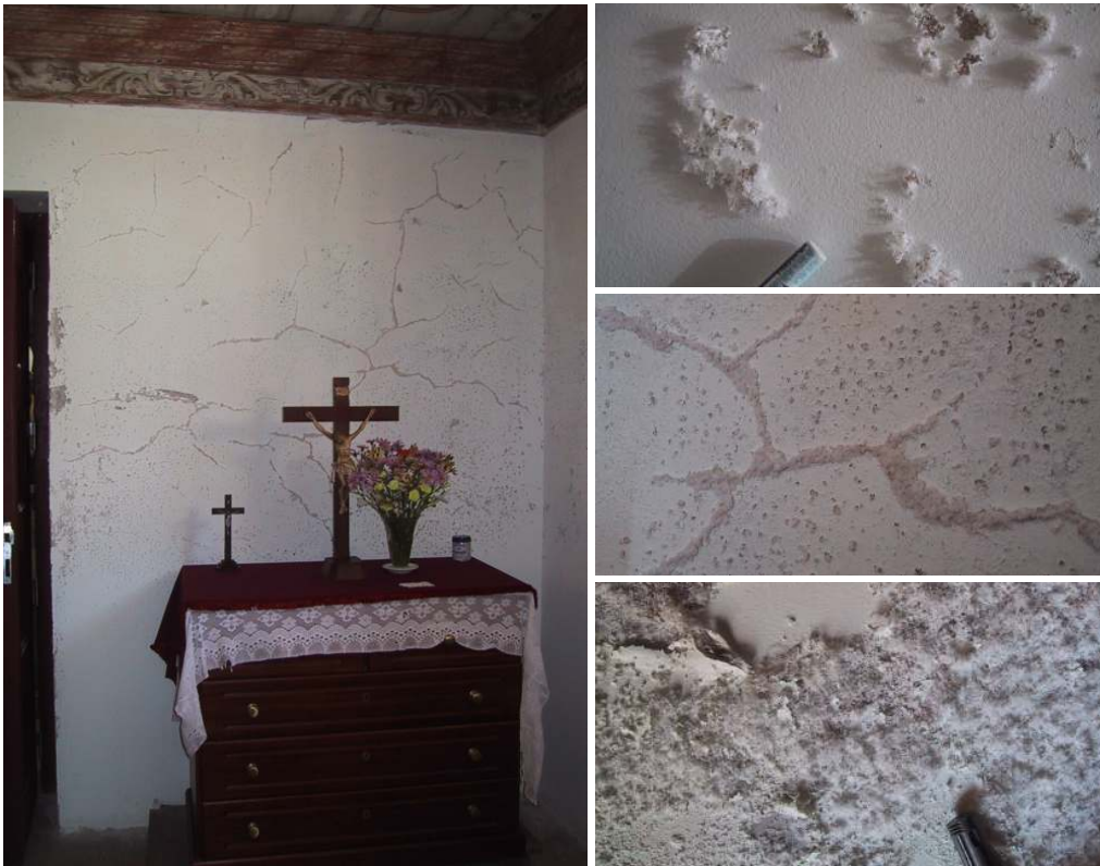
Fig. 6.12 – Extensive damage at the interior of Despacho House. On the left: cracking of the plaster/paint system and efflorescence is observed from around 70cm height from the pavement up to the top of the wall. On the right: damage details showing that salt crystallization at the plaster/paint interface causes rupture of the paint layer and further sanding of the underlying plaster (top), that efflorescence develops preferentially, though not only, on the cracks (centre) and that large areas are eventually covered with efflorescence (bottom).
