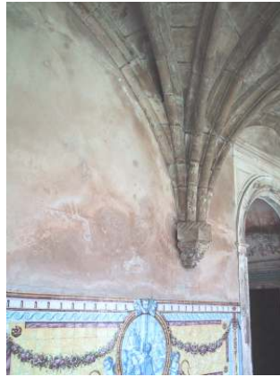
(b) Salt-damp – Cloister of Sta. Cruz Monastery, Coimbra, 2002
