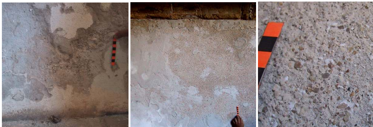
Fig. 6.15 – Sta. Clara: details of lower (on the left) and upper (on the centre) damage spots. Efflorescence agglomerations are observed on the upper spot (on the right)
