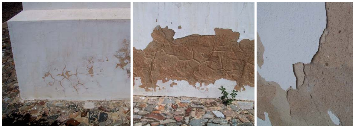
Fig. 6.5 – Salvas Chapel, damage spots on the SE façade. On the left: cracking of paint/render system and start of erosion, October 2003. On the centre; area in more advanced stage of degradation due to further sanding and crumbling of the paint/render system, October 2003. On the right; detachment of paint and of superficial coat of render, June 2002
