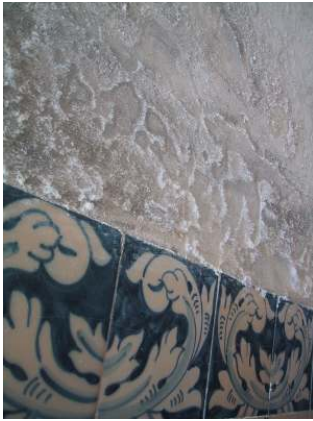
(a) Efflorescence – New See basement, Coimbra, 2003
