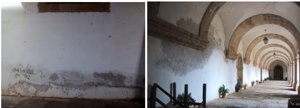
Fig. 6.14 – Sta. Clara: damage appears either close to the ground (NE wall, on the left) or higher on the walls, next to stone elements (NW wall, on the right).
