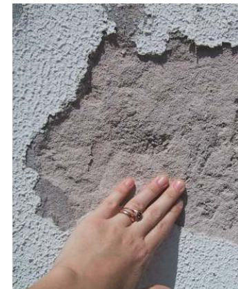
(i) Erosion – Arouca city hall library, 2002
