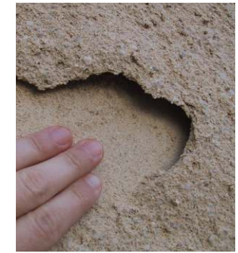
(f) Delamination (layering of material with laminated structure, in this case, a render applied in different coats) – Tibães Monastery, Braga, 2002
