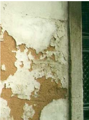
(d) Paint peeling – building in the historic centre of Santarém, 2003
