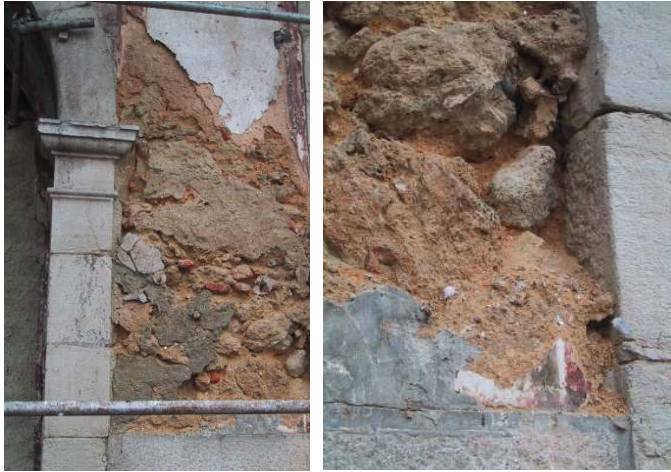
Fig. 6.22 – São Sebastião: masonry damage progresses as follows: (i) lime plasters and renders disappear due to progressive sanding and crumbling; cement repairs, apparently undamaged, detach; (ii) sanding and crumbling of the bedding mortar progresses on the exposed masonry, as seen in these pictures; (iii) fall of the stone elements eventually leads to masonry disintegration, as seen in the picture on the right.
