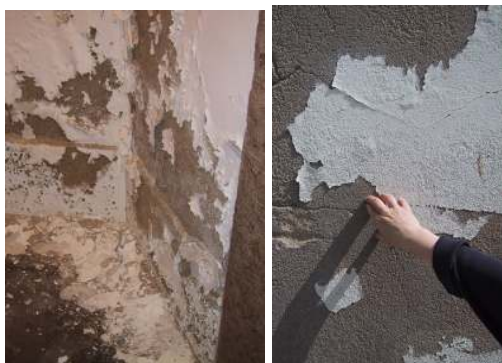
Fig. 5.39 – Paint damage arising without the presence of efflorescence: interior of Ajuda Palace, Lisbon (left) and exterior of building in Almada, Portugal (right).
