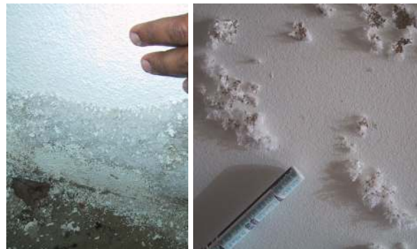
Fig. 5.40 – Paint damage by subflorescence pressure: Alhos-Vedros tide-mill (left) and interior of Despacho House, Pereira, Portugal (right).
