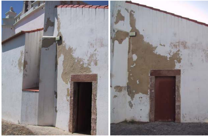
Fig. 6.2 - Salvas Chapel, NE (rear) façade: July 2002 (left), November 2003 (right)
