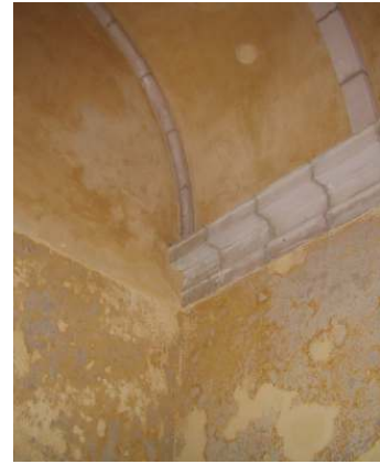
(c) Salt damp and staining – Alcobça Monastery, 2002
