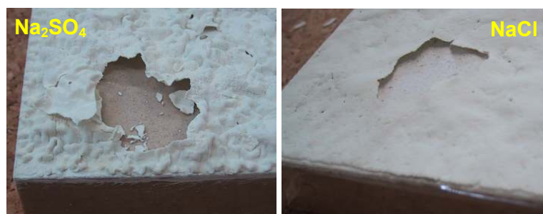
Fig. 5.38 - Damage to the acrylic paint during the second crystallization experiment: for sodium sulfate, after one hour soaking in the second cycle (left); for sodium chloride, at the end of the third cycle drying (right). The paint layers were intentionally perforated to allow observing the stone surface.
