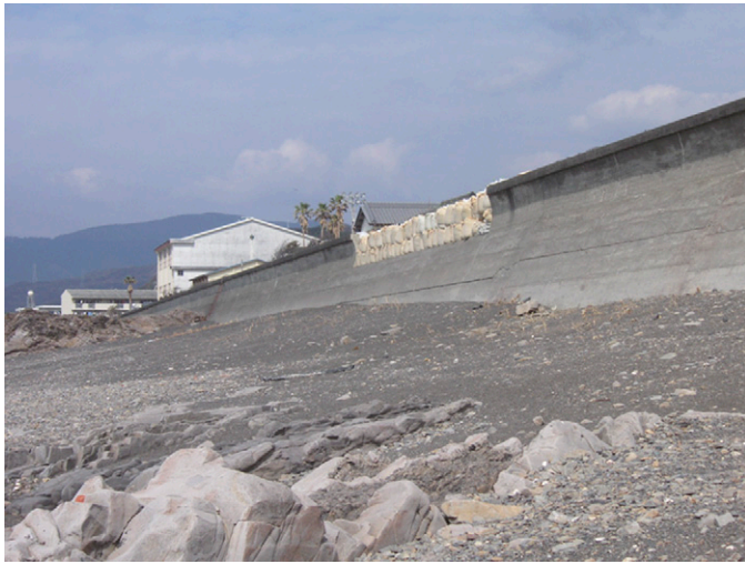
Fig. 3. View of the foreshore and seawall constructed on land (Nabae in Muroto City, Kochi Prefecture, Japan) (photograph by Hajime Mase)
