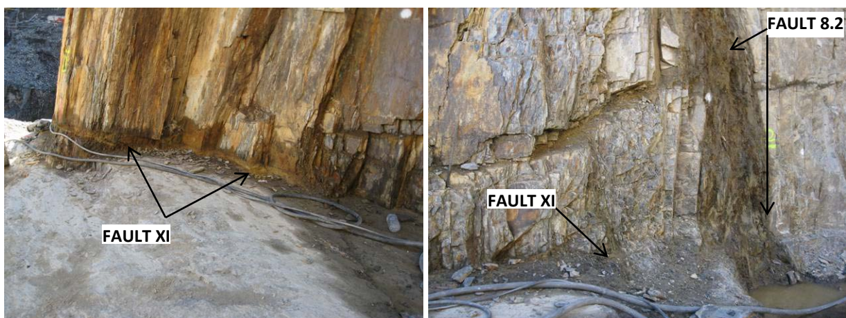
Figure 8 - Detail of discontinuities in the right abutment foundation
