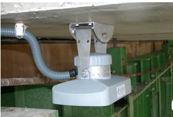
Fig. 8 – The radar level sensor
