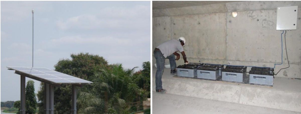
Fig. 11 – Photovoltaic panels and the batteries
