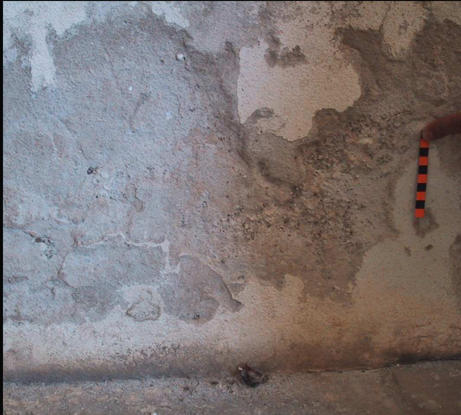
Damage close to the pavement
