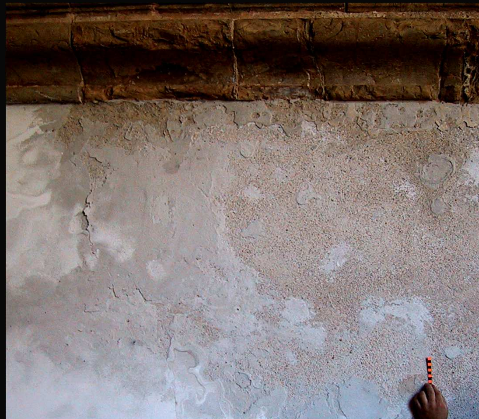
Damage up on the wall
