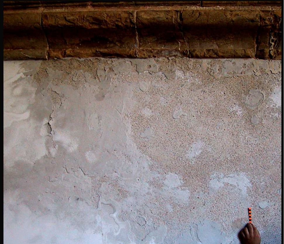
Damage up on the wall
