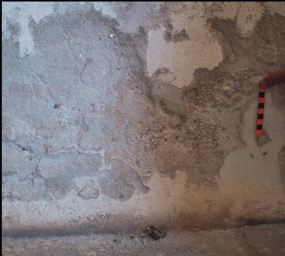
Damage close to the pavement
