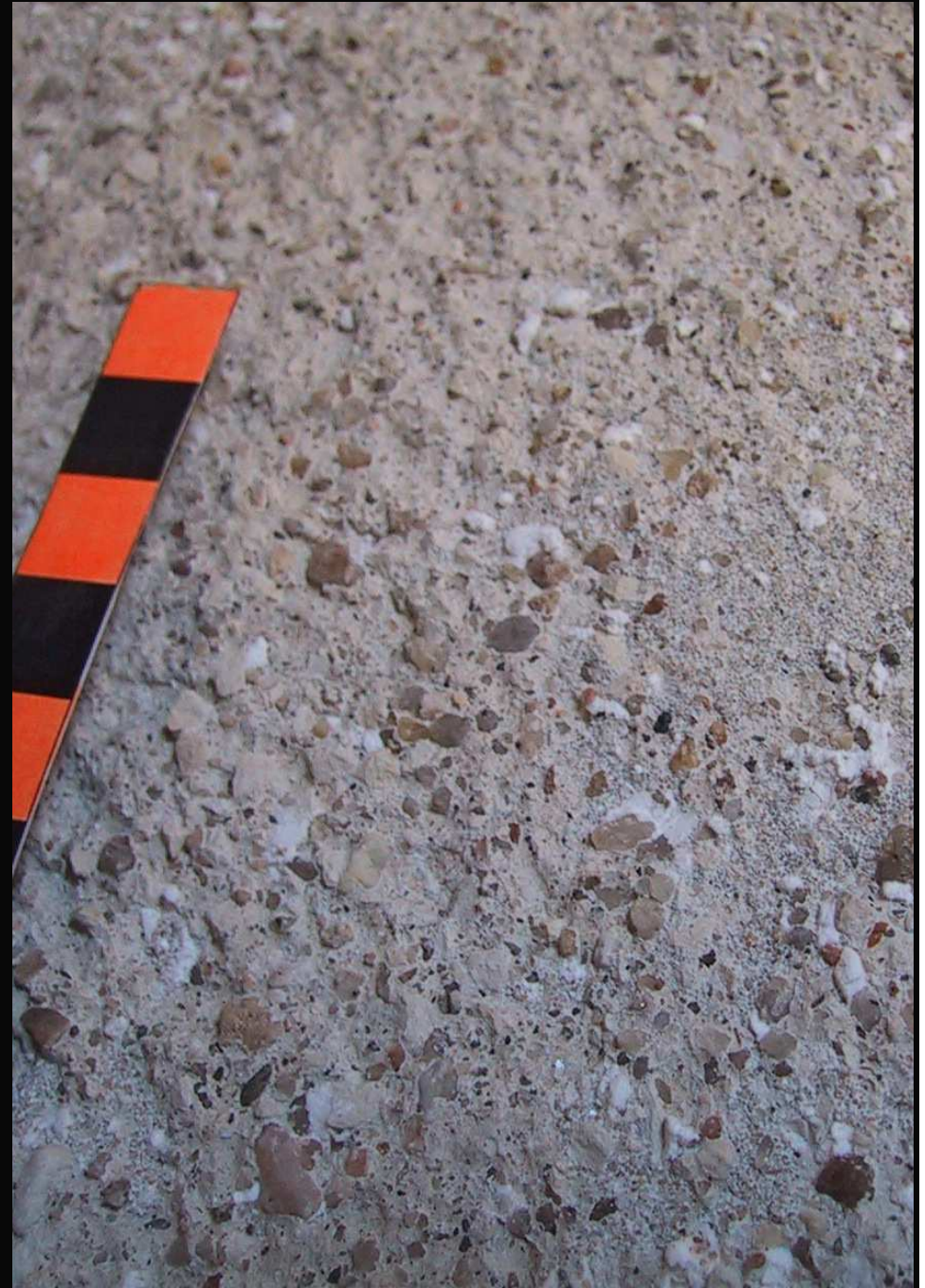
Damage up on the wall
