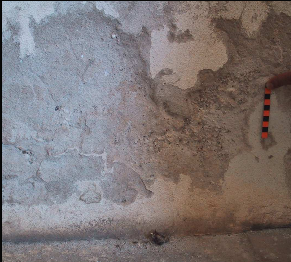
Damage close to the pavement
