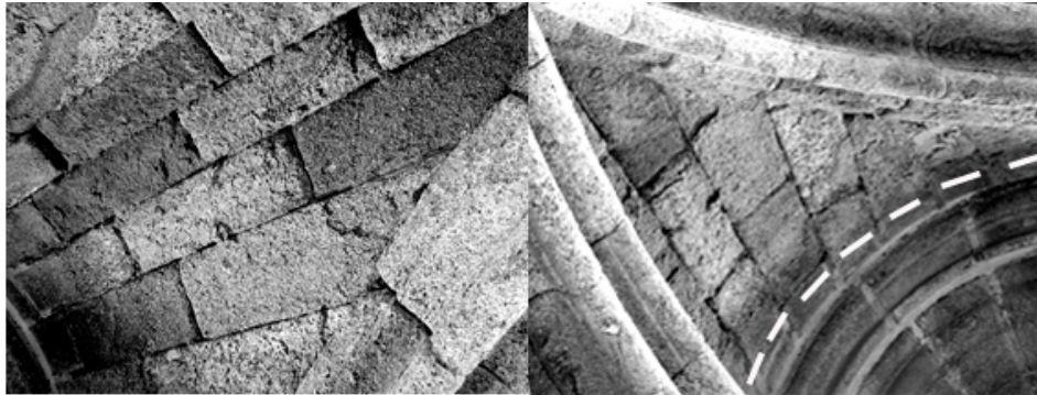
Figure 2. Extensive sand disintegration and erosion in the internal vault. The render is preserved on the right (zone delimited by dashed line).
