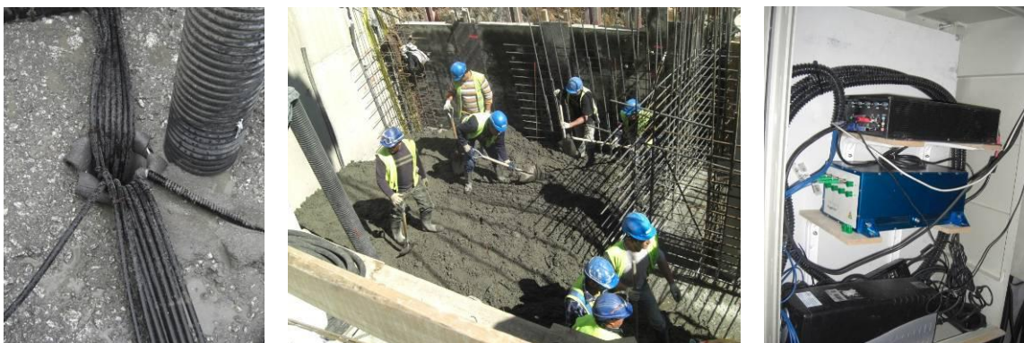
Figure 14 – Details of field installation: contrast between electrical cables and optical fiber conduct (left); concrete cast around sensors (center); fiber optic instrumentation acquisition point and respective equipment (right).
