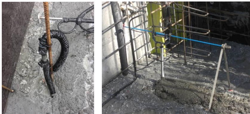
Figure 13 – Detail of the embedded temperature array (left), set up for joint meter gage (right).
