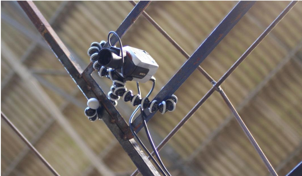
Figure 2 - COI1 flume. CATV Camera held in position using a “Joby GorillaPod® tripod” on the existing structure. Connected cable is BNC-terminated.
