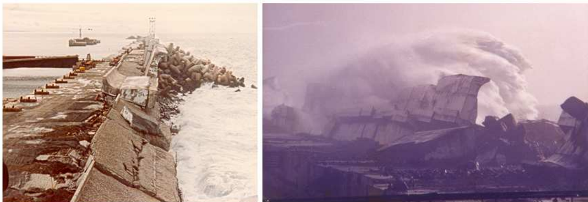
Figure 4: Port of Sines: failure of armour layer and superstructure
