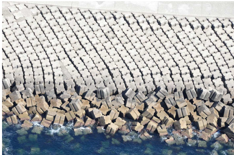
Figure 12: Sines West Breakwater: detail of Antifer placement at the upper part of the armour slope and at the crest berm
