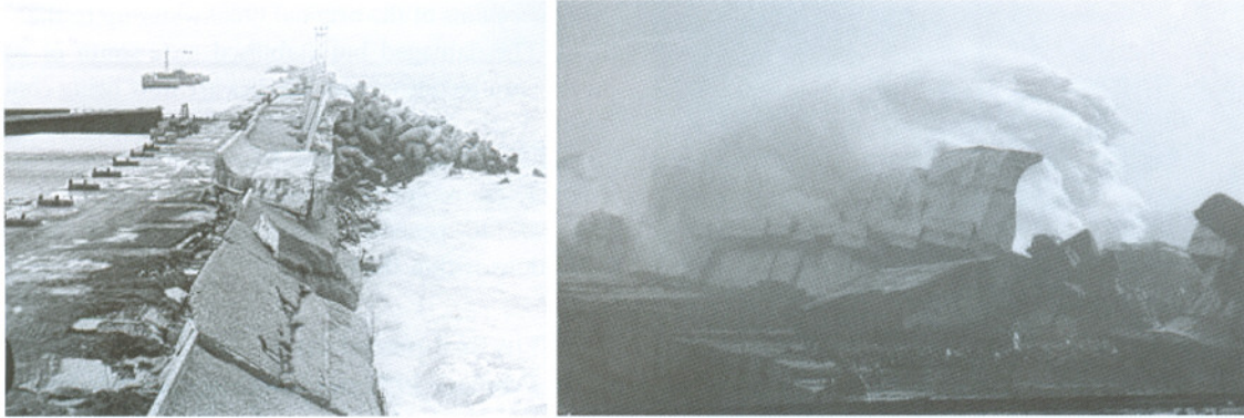
Figure 4. Port of Sines: failure of armour layer and superstructure
