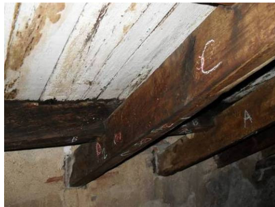
Figure 6 – Roof - Location of the roof beams where treatment and consolidation was conducted. (A) “low” degradation; (B) “high” degradation and (C) sound
