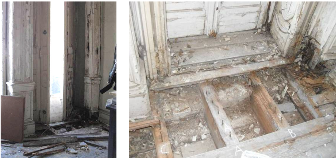
Figure 4 – Pavement1 – Location of the floor beams where treatment and consolidation was conducted.
