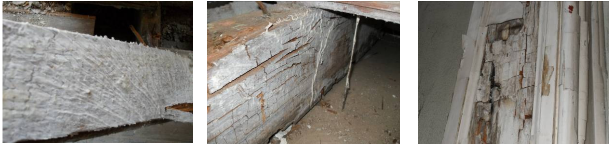
Figure 2 – Details of rotted timber in situ .
