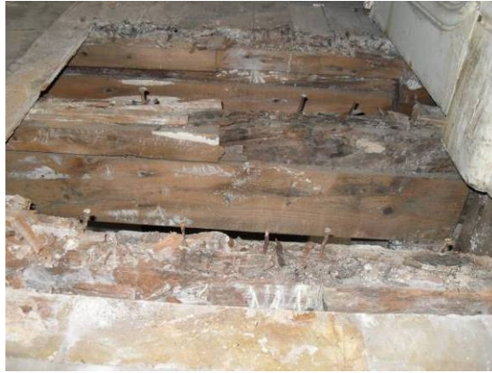
Figure 5 – Pavement2 - Location of the floor beams where treatment and consolidation was conducted.
