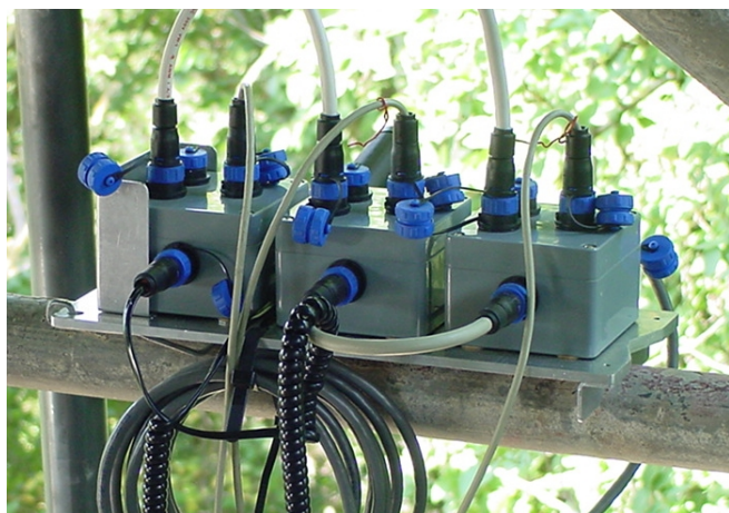
Figure 5 – Example of fixture of sensor boxes over the covering structure
