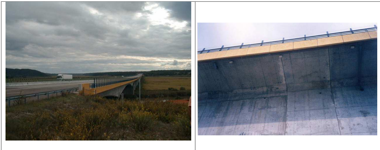
Figure 9 - A2, over Sado river valley. Runoff from this bridge is collected through plastic pipe to the structure at the base of the bridge and conducted to a major pipe. The discharge is made to river Sado, considering that the dilution factor is sufficient to eliminate significant impacts
