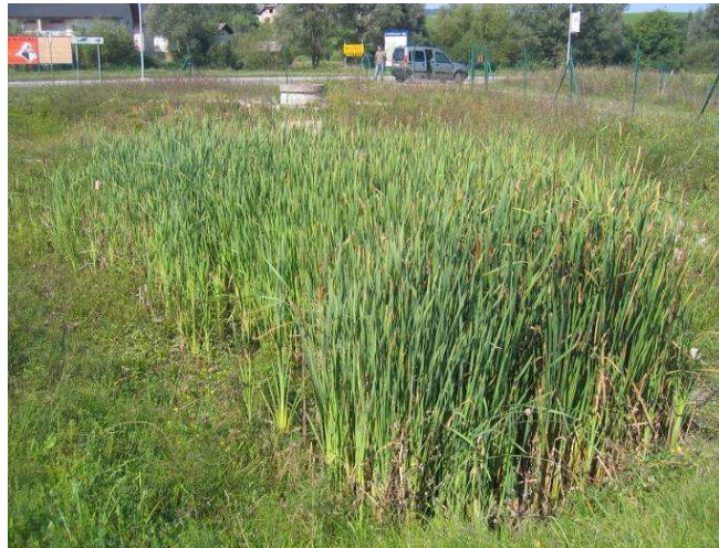
Figure 7 - Combination of mechanical and biological treatment with rush in artificial wetland – highway Ljubljana Ivančna gorica – central east Slovenia
