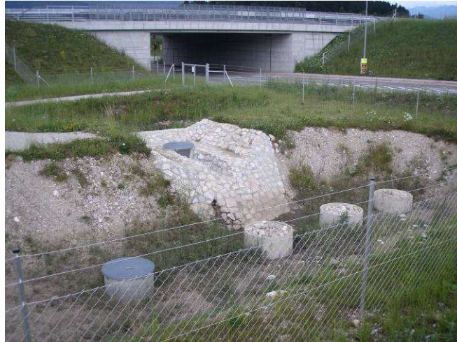
Figure 8 - Retention pond with infiltration pond and infiltration wells – highway Jesenice Kranj; Northwest Slovenia
