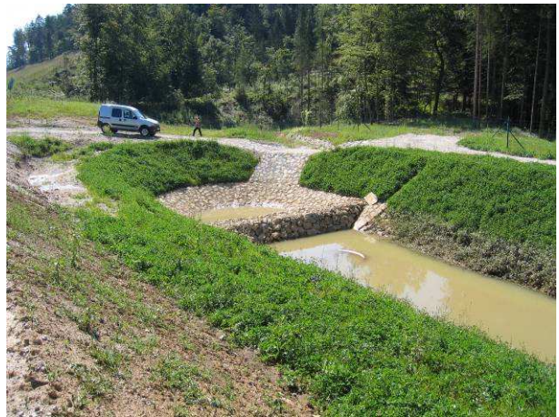
Figure 5 - Ground retention pond with sedimentation pond and spillway along the highway Ivančna gorica – Novo mesto Southeast Slovenia
