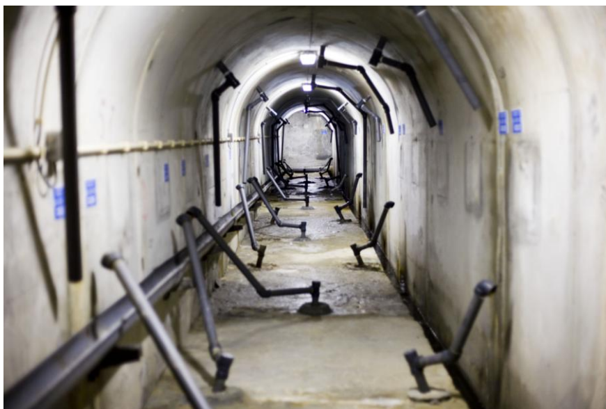
Figure 4.43 – Top of the extension of the downstream drainage gallery towards the right bank.
