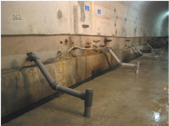
Drainage boreholes in the gallery of a concrete dam. The grout holes were drilled from the gutter, which is filled with water, as shown in the photo.
